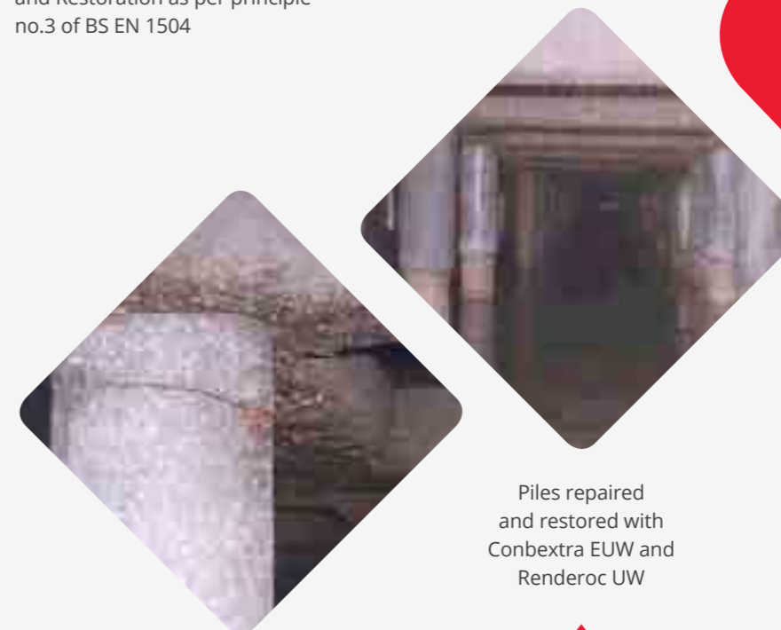
Cracks in the Jetty piles
