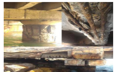
Severely spalled and distressed structural members (underside of the berth)
