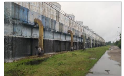
Condition of IDCT cooling towers before repair
