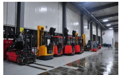
Charging area for electronic Fork trucks
